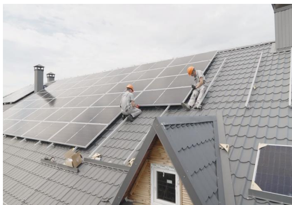
Figure 4-1-2. PV project at Liceym Mriya, Irpin
