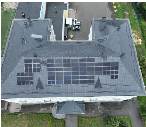
Figure 4-2-1. PV project at Chernihiv school No. 3
