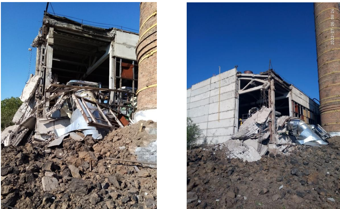
Figure 5-1 Consequences of the bombing of one of the boiler houses...
