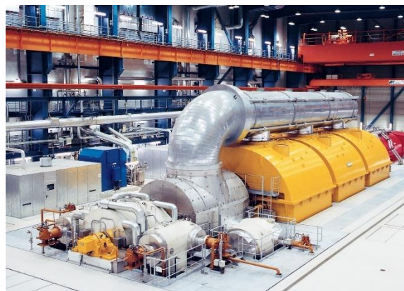
Figure 6-3 An illustration of a general view of turbogenerator
