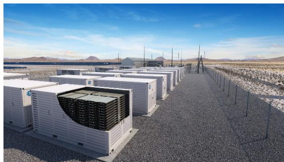
Figure 6-6 An example of industrial energy storage
